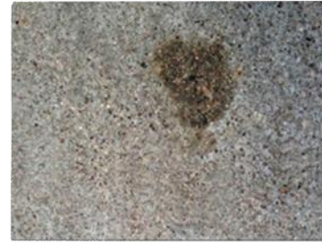
Oil on concrete before treatment
